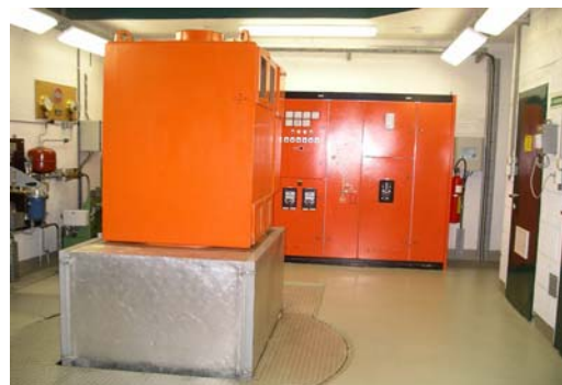
Generator, Sagfossen, Siljan
